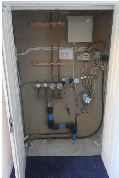
Back of services cupboard
